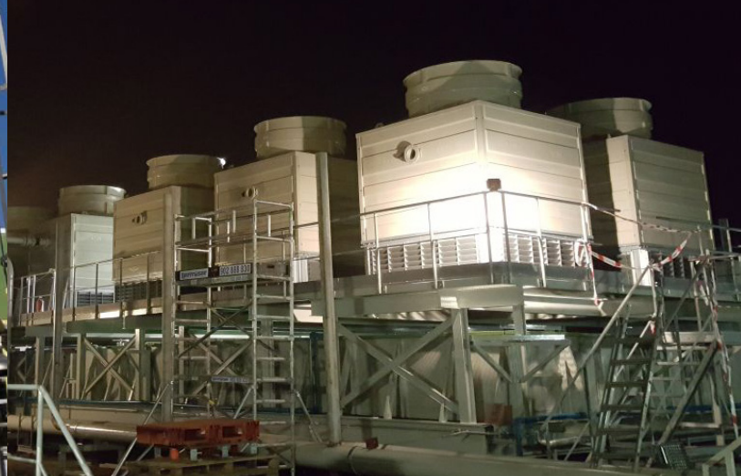
MALL EL CORTE INGLES - (GRAN VIA, BILBAO) AIR CONDITIONING - 12 X 1,050 KW
