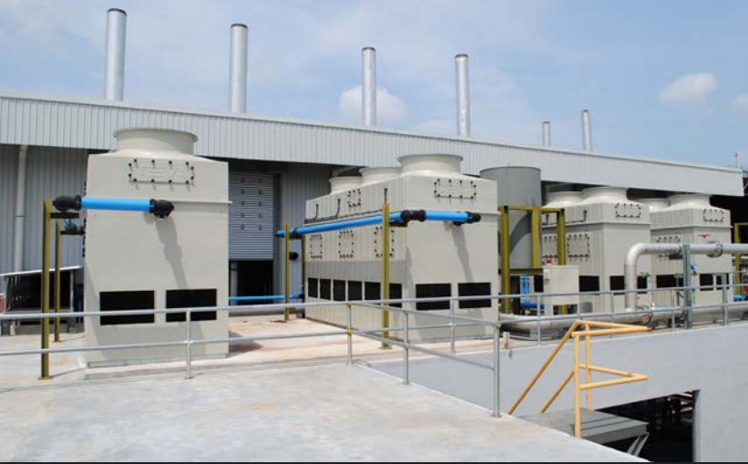
AUTOCLAVE (MALASIA) 4 TOWERS WITH A TOTAL OF 8,000 KW
